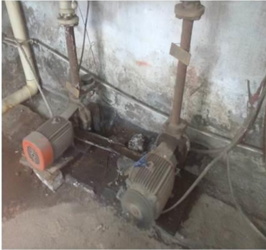
Old inefficient monoblock pump
